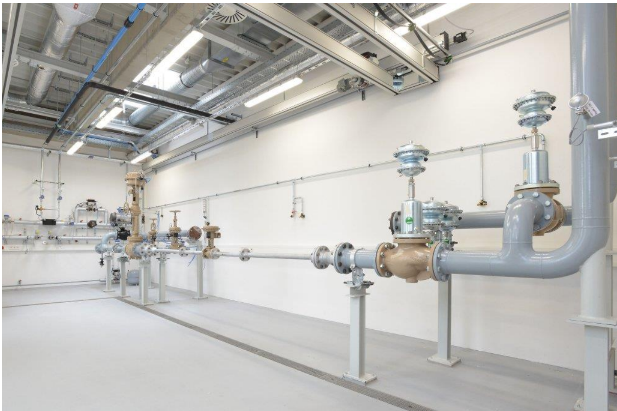
Abb. 6: Flowlab: District Energy © SAMSON AG
